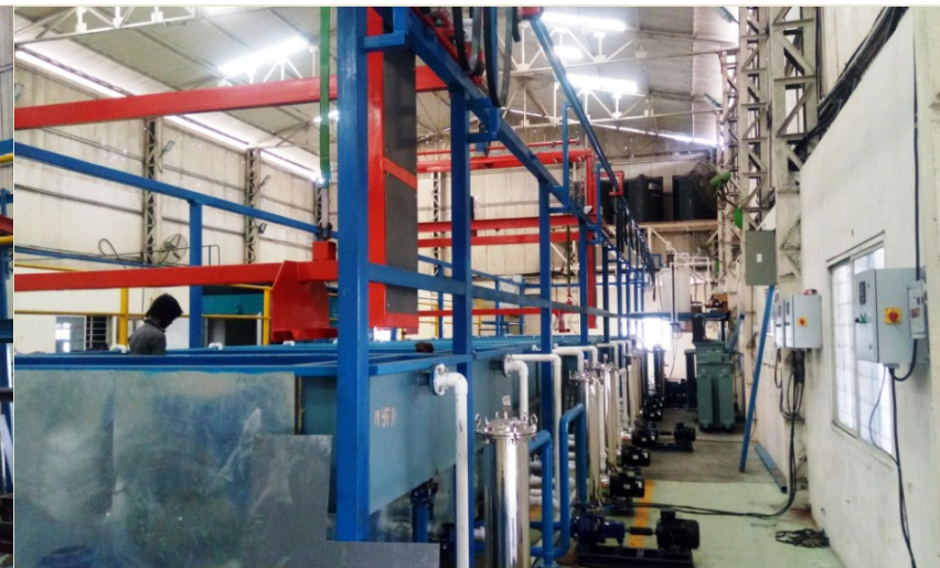
CED COATING PLANT, PUNE
