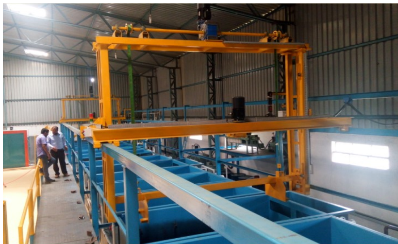
CED COATING PLANT, PUNE
