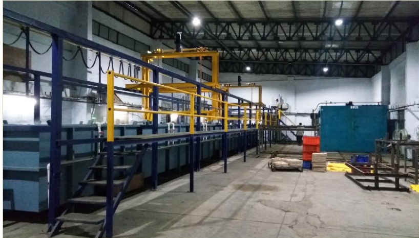
CED COATING PLANT, KOLHAPUR
