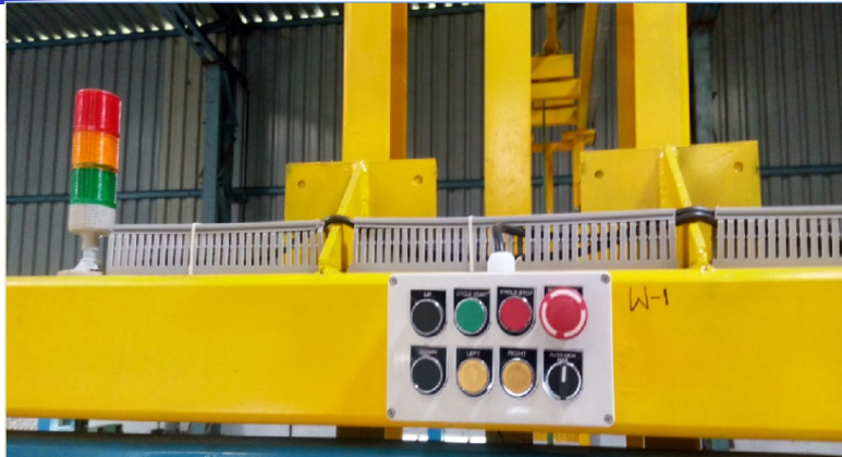
OPERATOR BOX & TOWER LAMP
