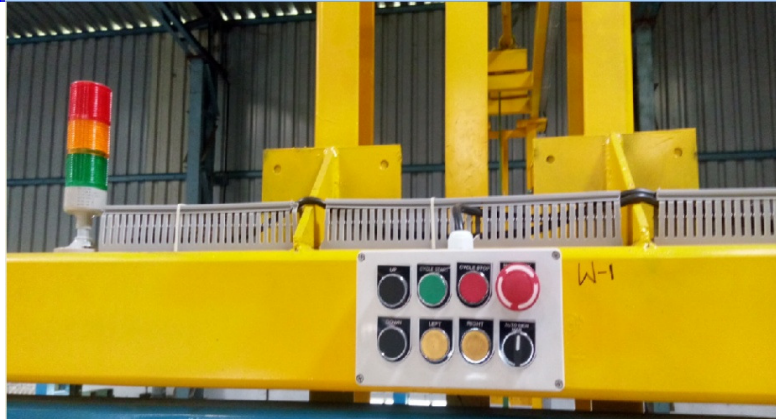
OPERATOR BOX & TOWER LAMP
