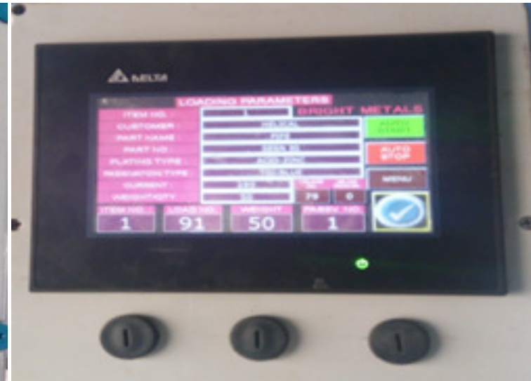
OPERATOR HMI CONSOLE
