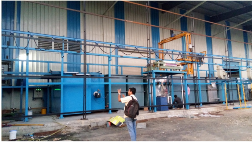
PHOSPHATING PLANT, NAGPUR
