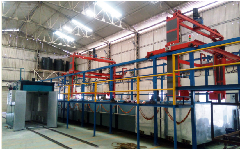
CED COATING PLANT, PUNE
