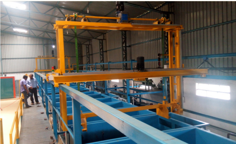
CED COATING PLANT, PUNE
