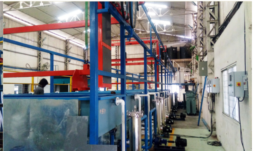
CED COATING PLANT, PUNE
